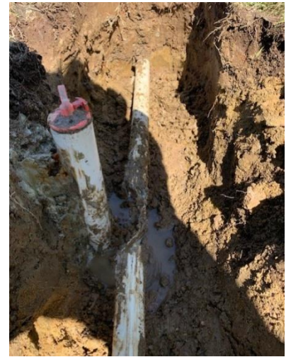
Irrigation damage at Founders Park.
