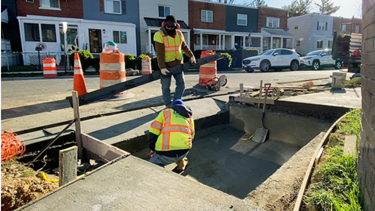
A crew from D&F Construction works on a project to increase inlet capacity on Manning Street on April 16. (City of Alexandria)
