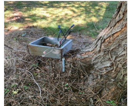
Electrical box/wires secured at Fort Ward Park before.
