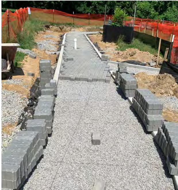
Permeable pavement BMP under construction at the Fort Ward picnic shelter pathway
