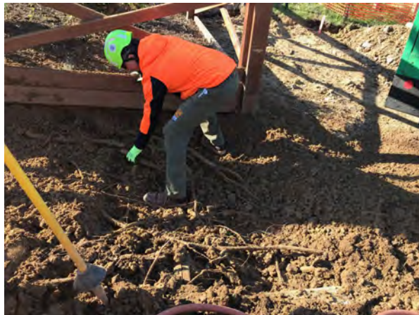
Air spading may be used to loosen compacted soil, to expose tree roots, and to keep critical root systems intact. This application was used for construction of a sidewalk at Ewald Park.
