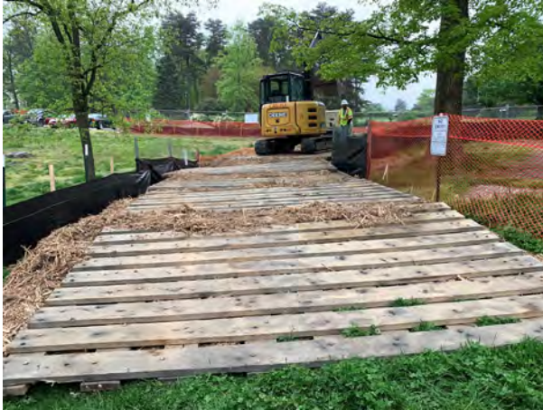
Tree mats were used for equipment access during construction of the Fort Ward picnic shelter pathway
