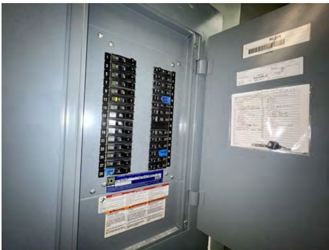
33. Circuit breaker panel
