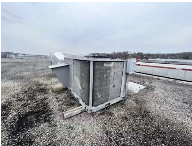
27. Packaged rooftop unit
