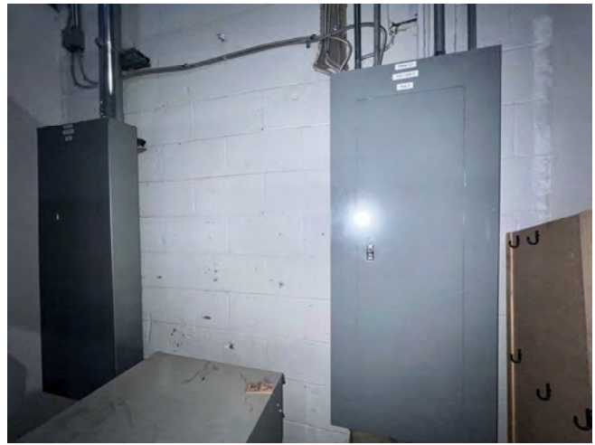
32. Main distribution panel
