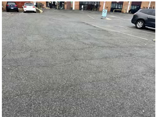
10. Cracking in asphalt pavement
