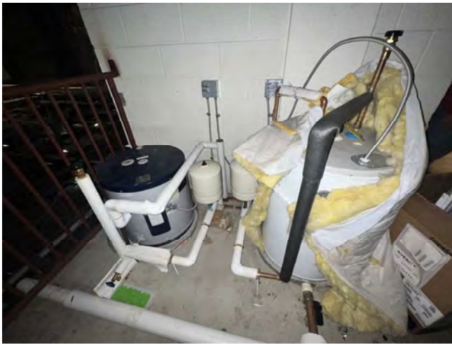
25. Hot water heaters
