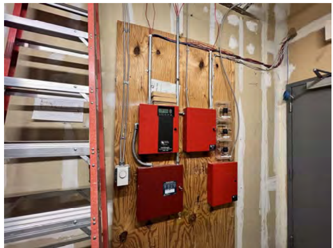
34. Fire alarm control panel
