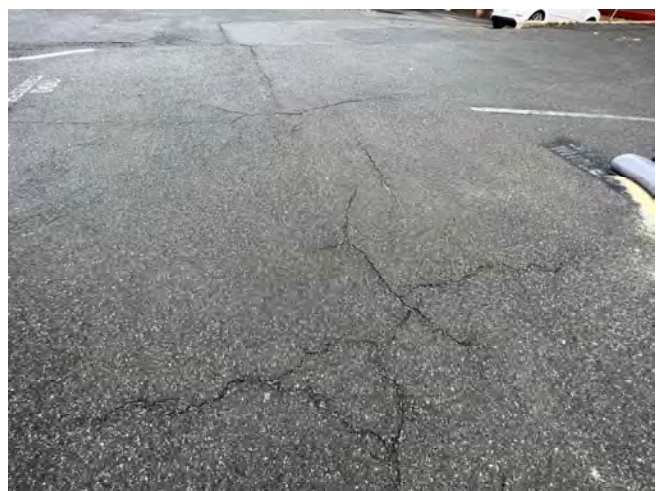
12. Cracking in asphalt pavement
