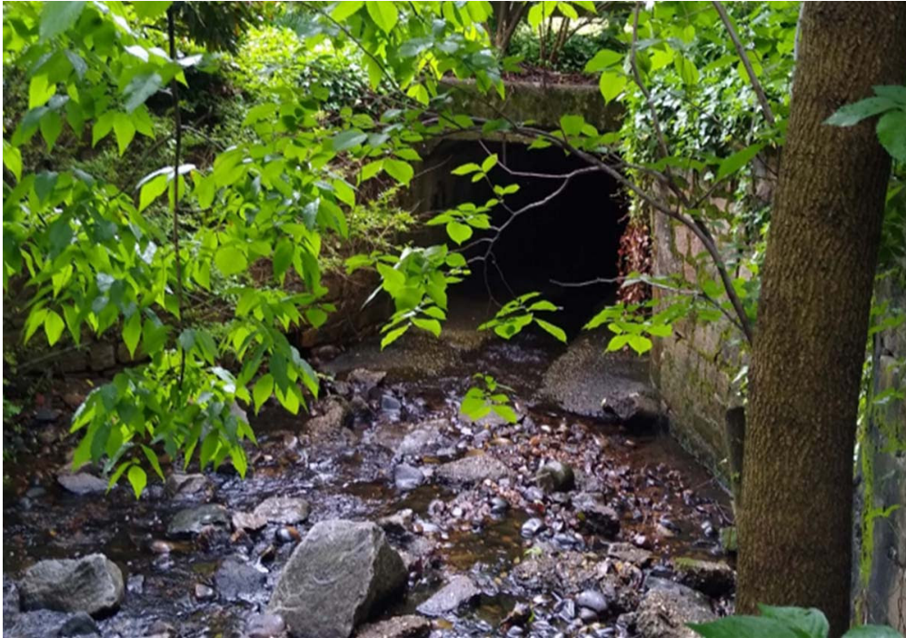
Existing Hooffs Run culvert opening near W. Glendale Ave. and Junior St.
