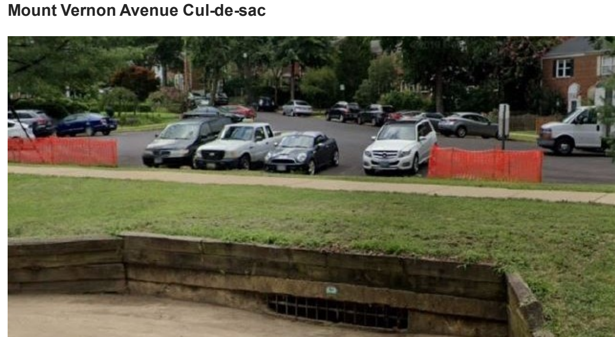
Construction on Mount Vernon Avenue is expected to begin in Spring 2024 to address flooding concerns. The project will mitigate flooding for odd-numbered townhomes on the south end of Mount Vernon Avenue. (City of Alexandria)
